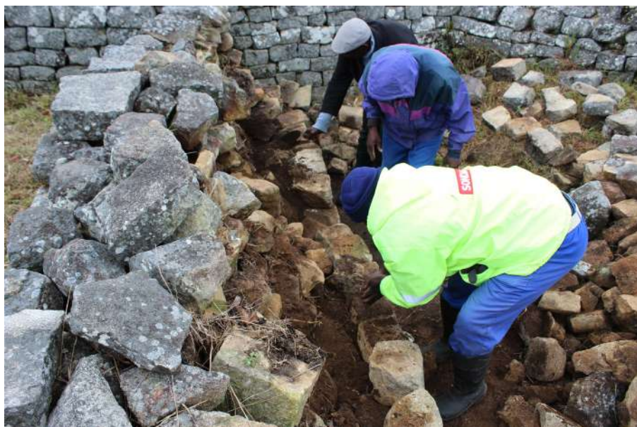
Figure 5.7 Stonemasons employing traditional skills to reconstruct collapsed walls at Great Zimbabwe (Source: NMMZ, 2018).
