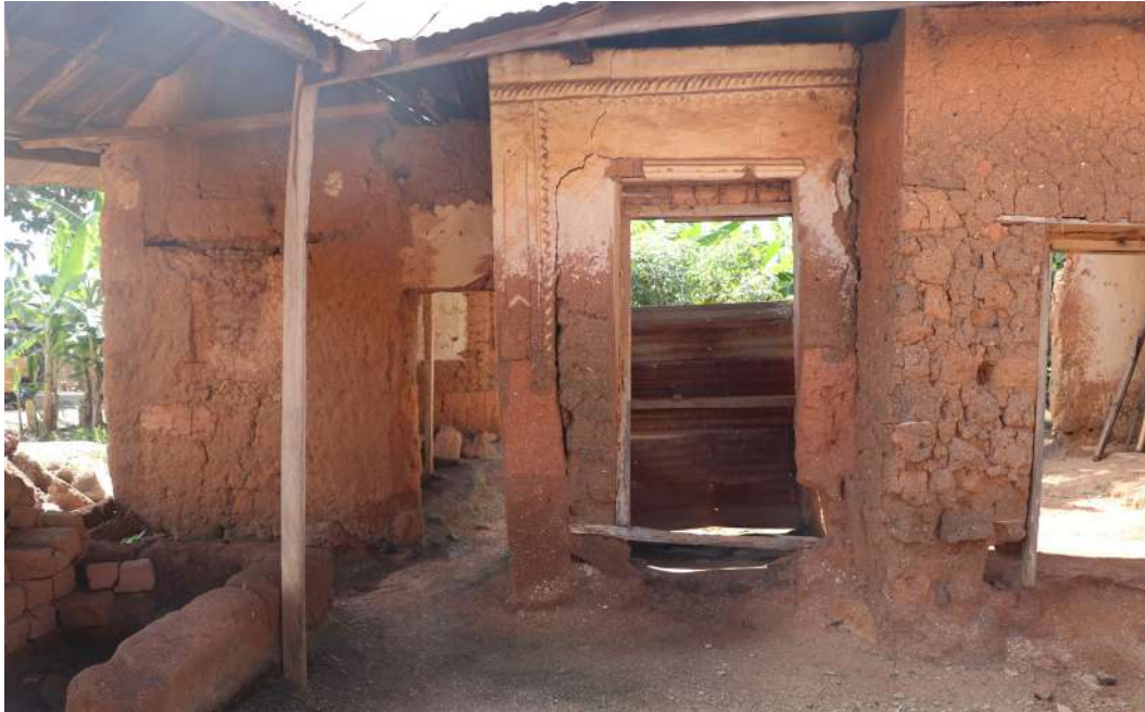
Figure 3.6 Impacts of climate change on the Asante Traditional Buildings (Source: Chris Wetcher, 2019).
