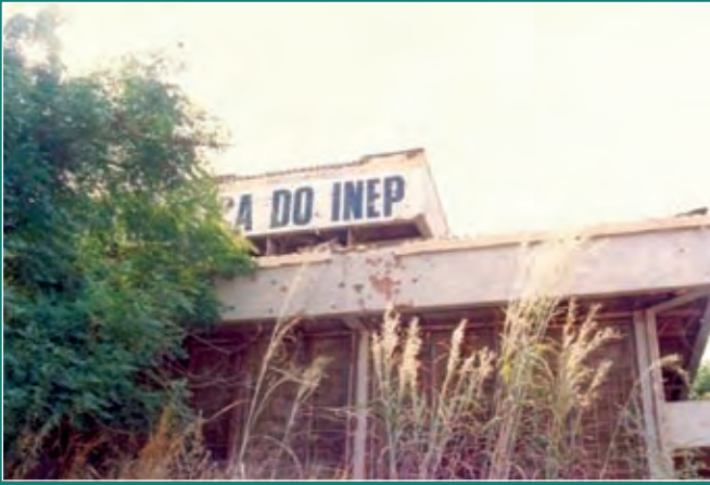
FIGURE 62 Building of the National Institute of Studies and Research (INEP) in Conakry, Guinea-Bissau, after occupation by the military and subsequent abandonment.
