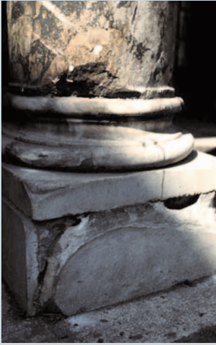
1 Marble deterioration due to sulphates (page 3)
