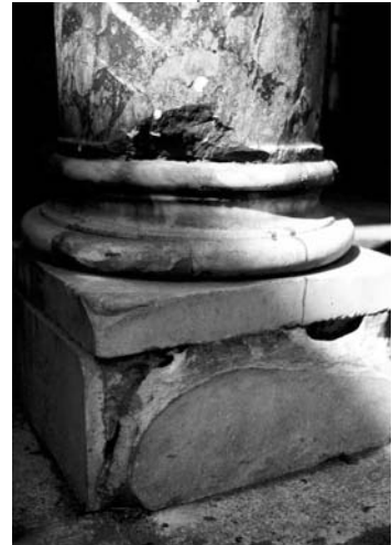
1 Marble deterioration due to sulphates colour print on inside back cover
