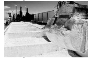
7. Lime putty pits
