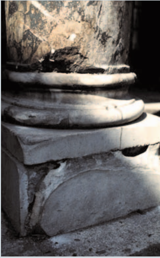
1 Marble deterioration due to sulphates (page 3)
