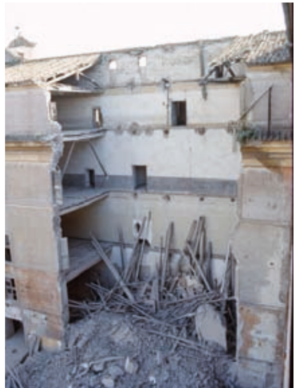
FIGURE 4-5 Collapse of part of the San Michele building, 1 April 1977
