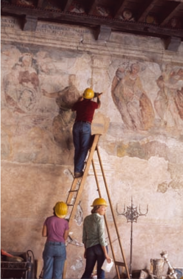
FIGURE 5-19 Mural paintings course in Venzone (Friuli), restoring the wall paintings of the Town Hall, 1976
