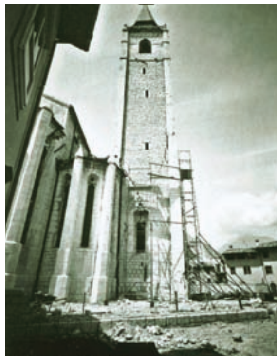
FIGURE 4-26 Friuli earthquake, Venzone cathedral; photogrammetric record by ICCROM-Austrian team after first quake
